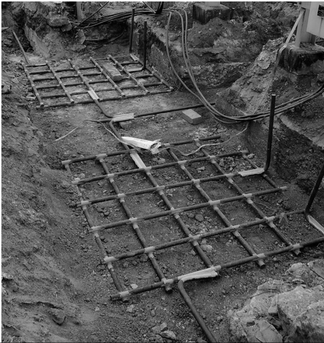
Earth Mat in 110kV side of a 220/110 kV Substation
